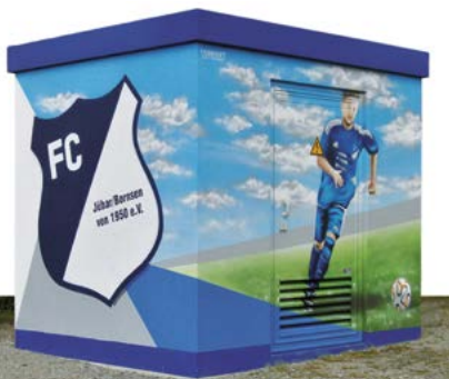
Designed substations Left: in Jübar Right: in Lehmke
