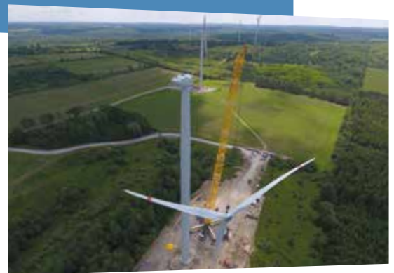
wpd Sumac Ridge wind farm during completion of turbine installation at the end of 2017.
